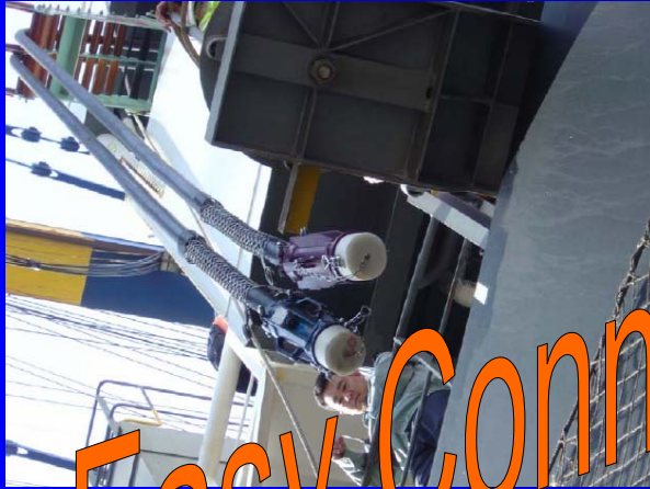
High voltage cable
